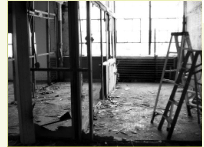
A work in progress, Isles' Mill One at One Johnston Avenue is slated for completion in late 2010.
